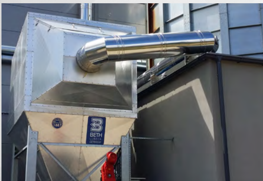
Elektrofiltr spalin / An flue gas electrostatic precipitator
